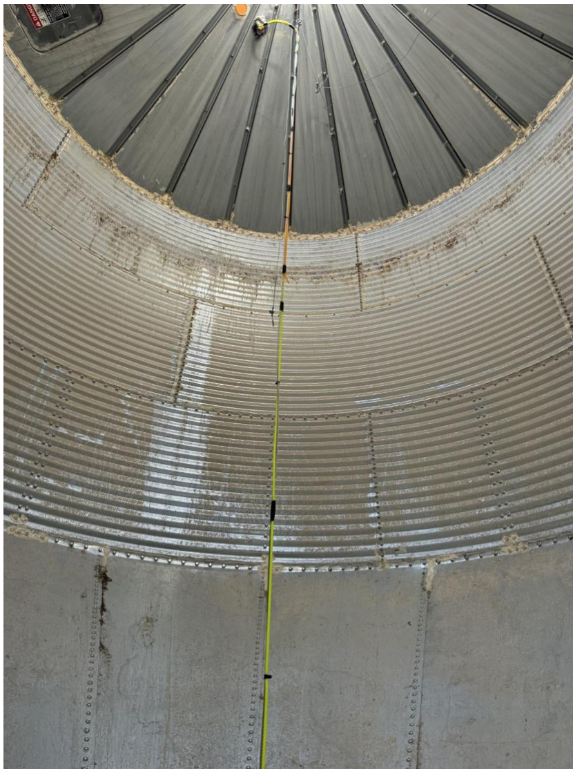
Figure 3. Cables inside the bin.
